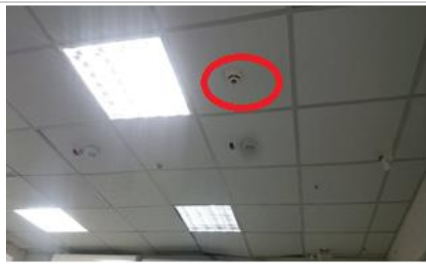
The Automatic Fire Alarm Sensor System
