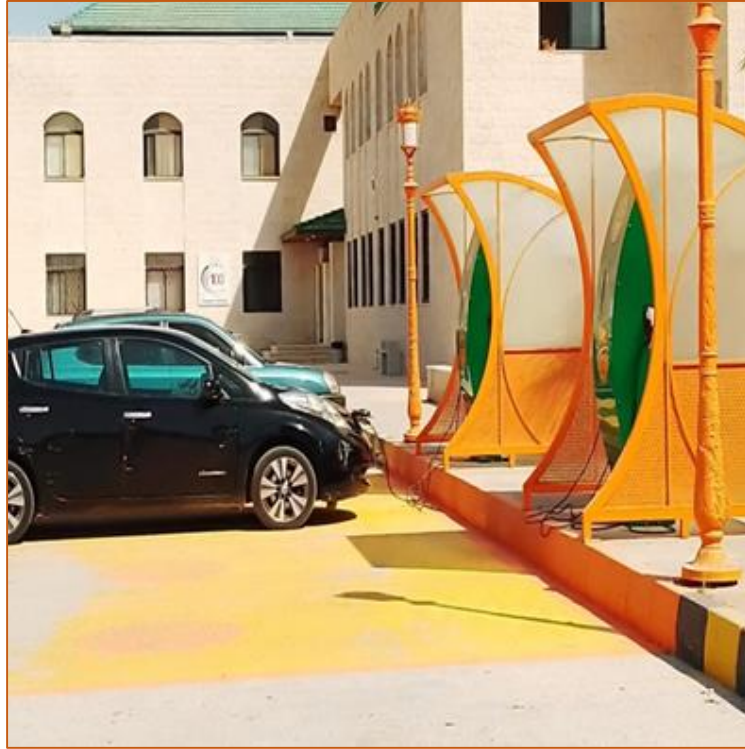
Electronic Cars Charging Stations (ECCS)
