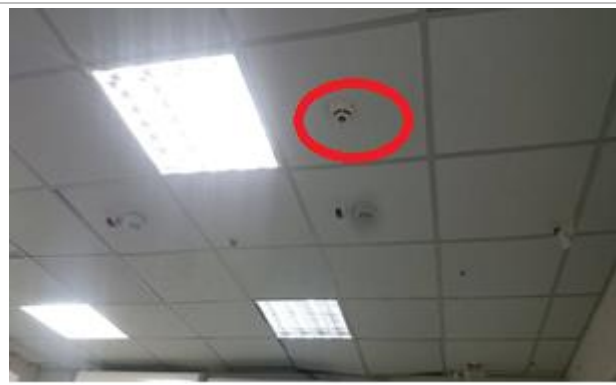
The Automatic Fire Alarm Sensor System
