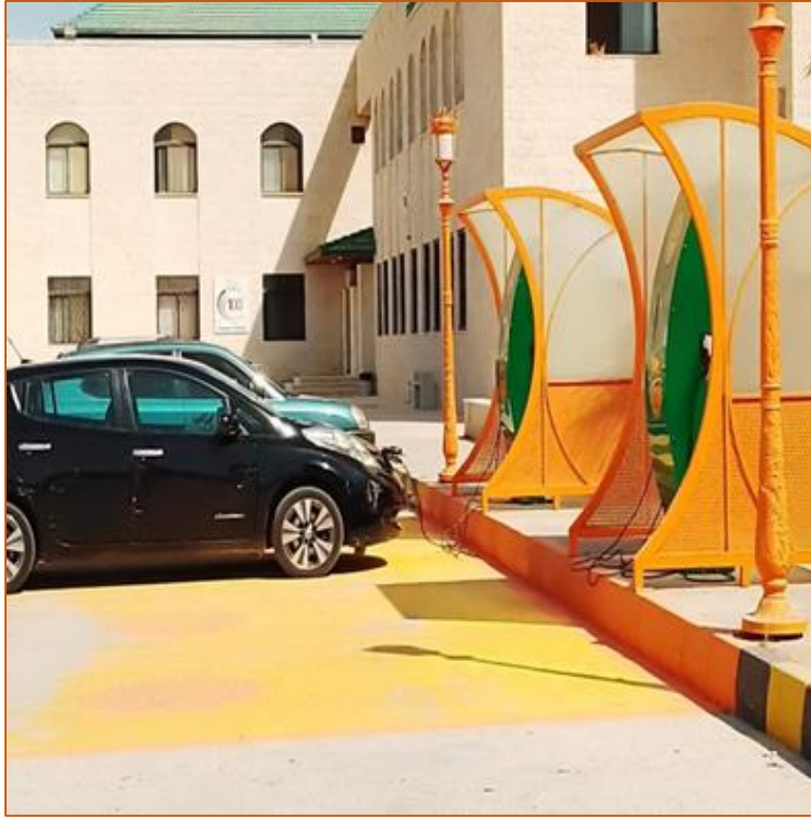
Electronic Cars Charging Stations (ECCS)
