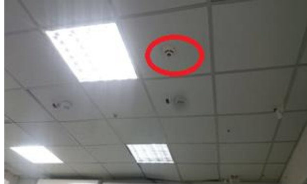
The Automatic Fire Alarm Sensor System
