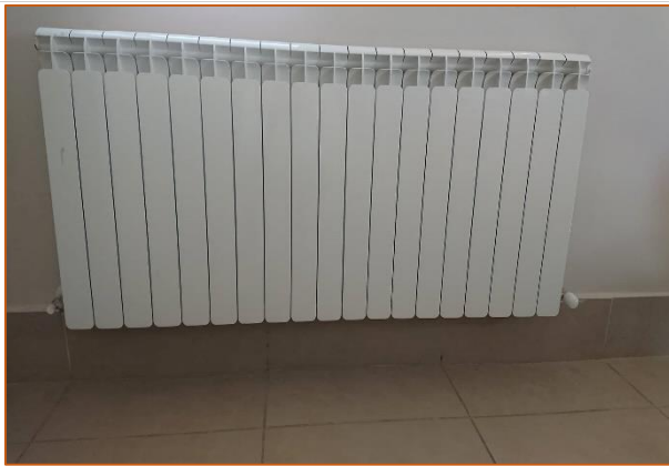
The Automatic heating System
