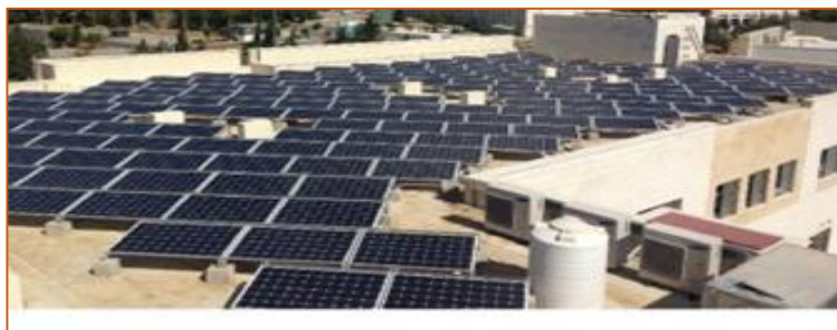
University Solar Photovoltaic (USVP)
