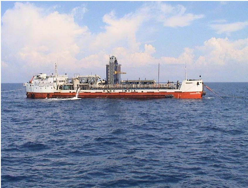
Fig. 9.10. A view of barge-mounted desalination plant off Tuticorin coast, south India.
