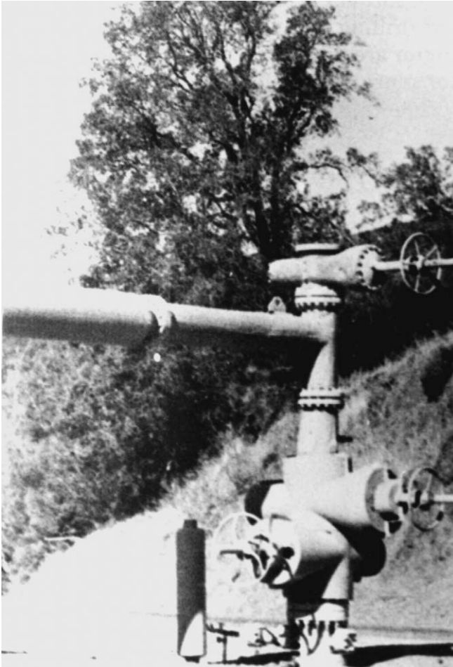
Fig. 7.16. A typical valve tree at Cerro Prieto (photograph by HG).
