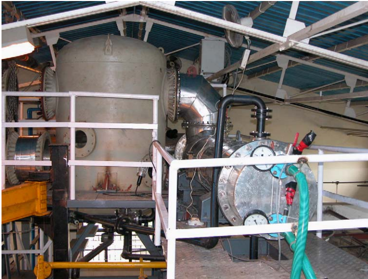
Fig. 9.2. A 5,000 l per day capacity plant commissioned at NIOT (Kathirola et al., 2006).
