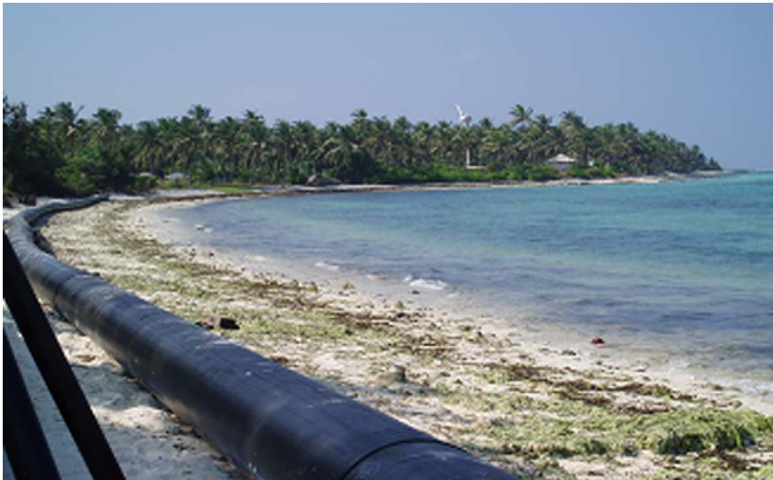
Fig. 9.6. View of the 600 m long HDPE pipeline used to bring cold water up to the plant site.
