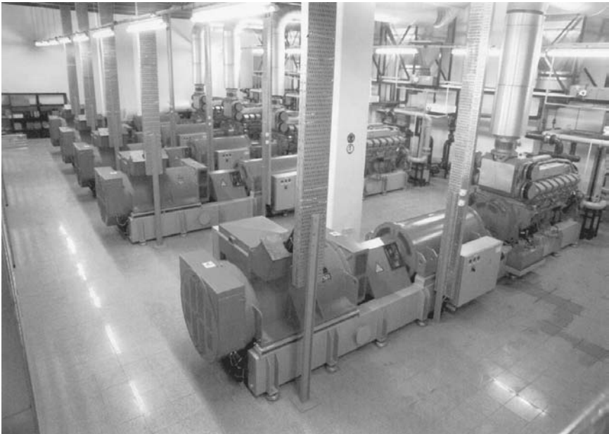
Figure 6.15 Typical machine room for a large computer system.
