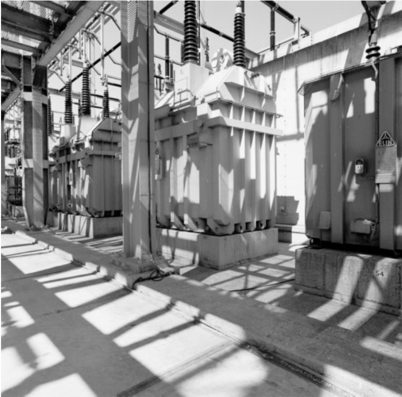
Figure 10.8 Short-circuit transformers. (courtesy of KEMA)
