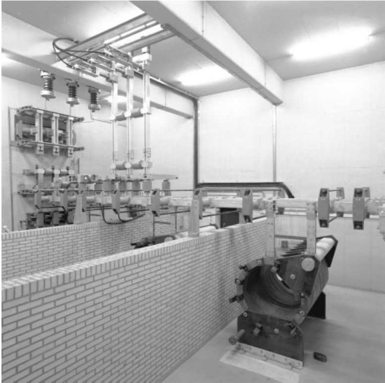
Figure 10.7 Current limiting reactors for one short-circuit generator. (courtesy of KEMA)
