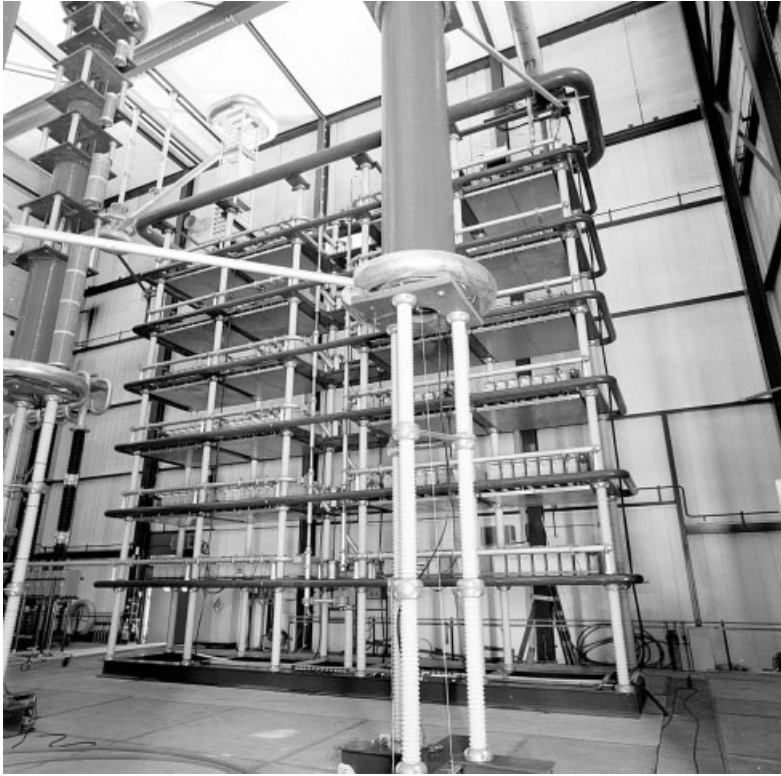
Figure 10.17 Main capacitor bank C_0 and main inductance L_1 of KEMA's synthetic test facility (courtesy of KEMA)
