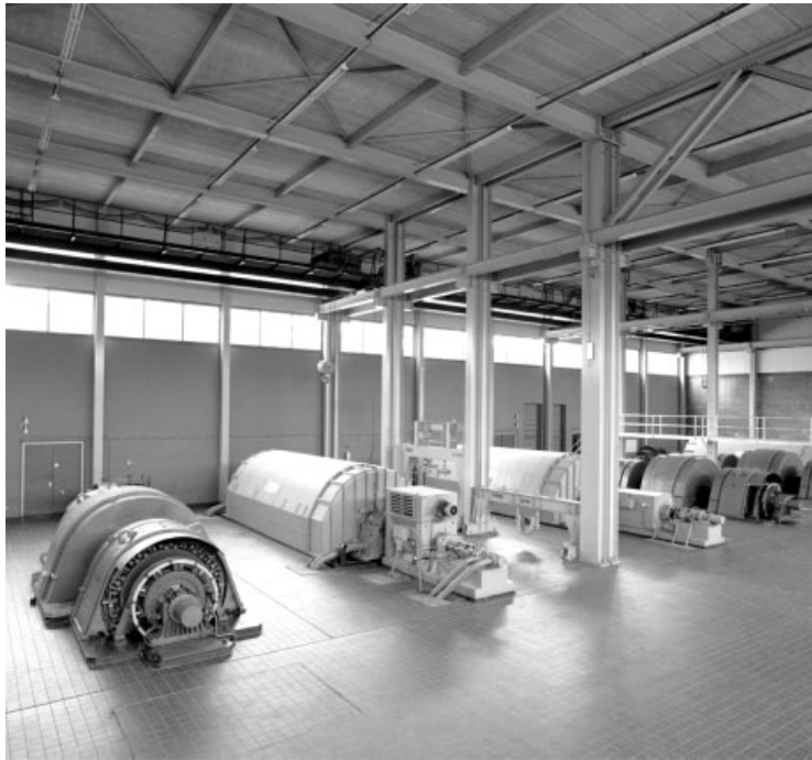
Figure 10.4 Two of the four short-circuit generators with their auxiliary machines in KEMA's generator room (courtesy of KEMA)
