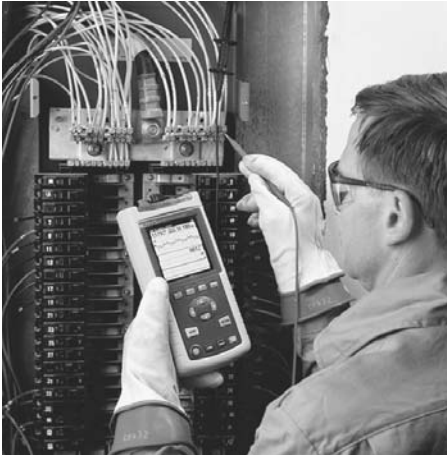
Figure 7.13 Typical service entrance panel. (Reproduced with permission of Fluke Corp. ©.)
