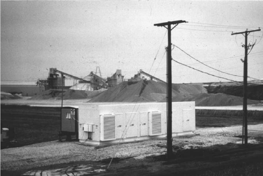
Figure 4.26 DSTATCOM installation. (Courtesy of EPRI.)
