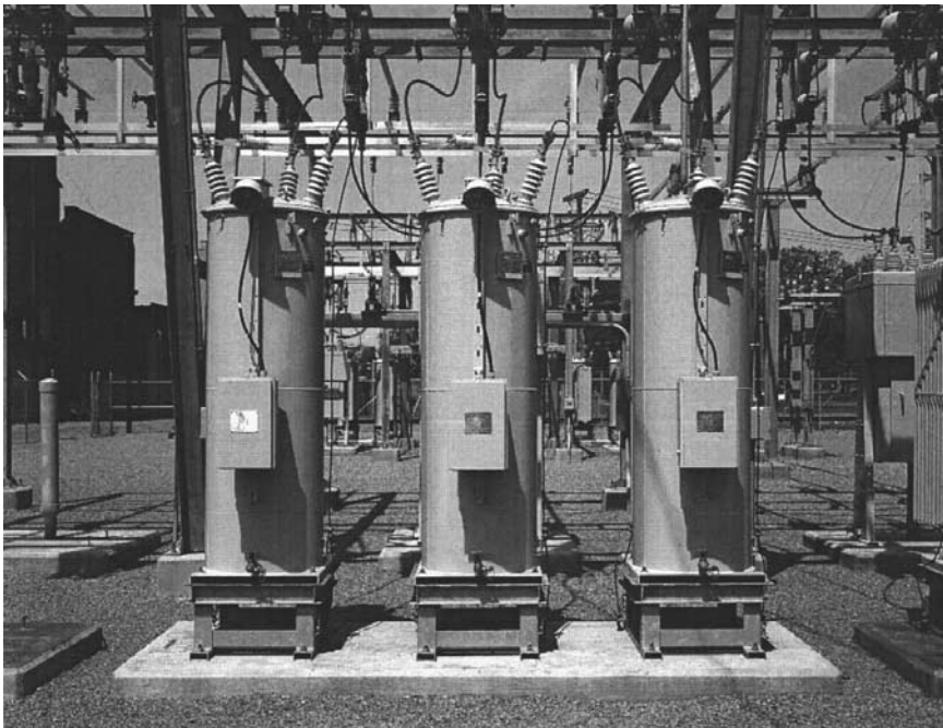
Figure 7.7 Typical utility three-phase 32-step voltage regulator bank. (Courtesy of Cooper Power Systems.)
