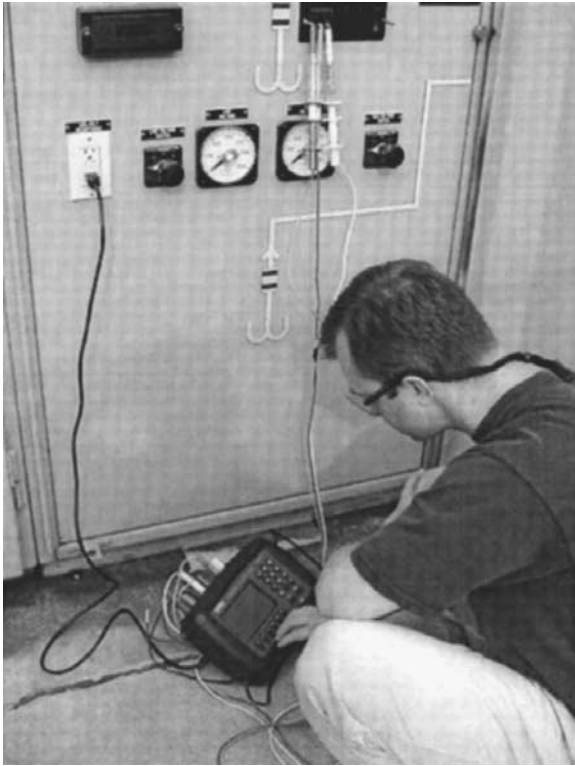
Figure 11.11 Demonstrating the use of a hand-held, three-phase power quality monitoring instrument to quickly evaluate voltages at the mains.
