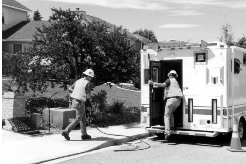
Figure 10.8. A fiber-to-the-home/PON installation in Wenatchee, Washington. [Credit: The Light Brigade.]
