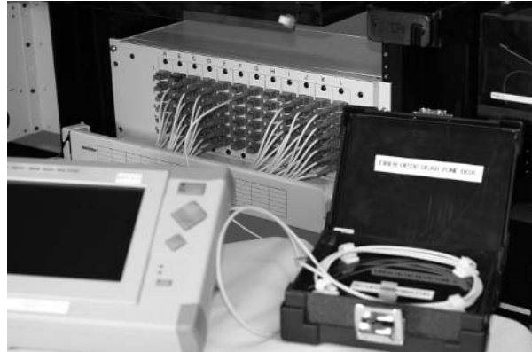
Figure 3.3. Typical mini-OTDR linked to a fiber-optic patch panel. [Credit: The Light Brigade.]
