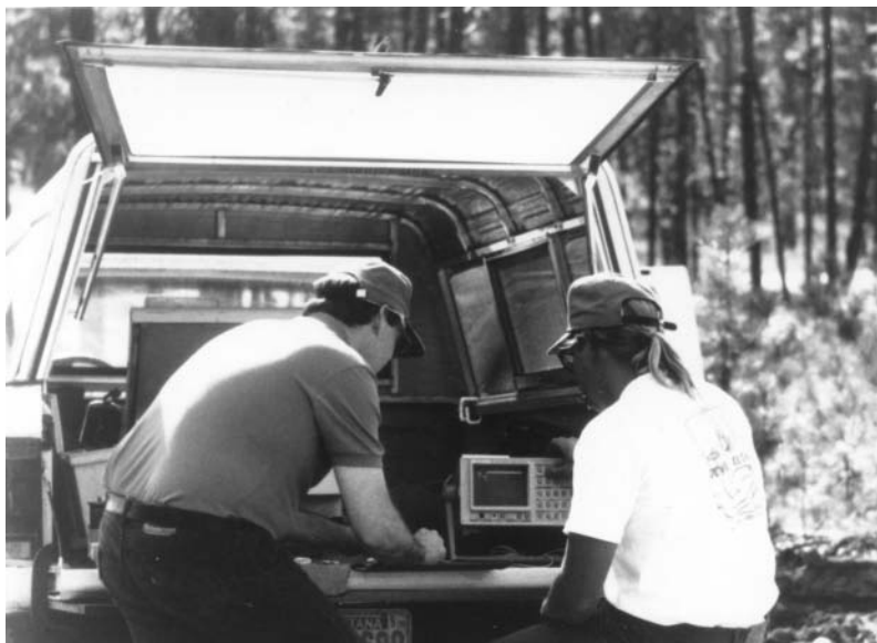
Figure 15.1. Acceptance testing optical-power ground wire with an OTDR. [Credit: The Light Brigade.]
