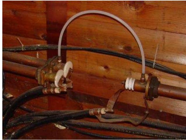
Figure 14.52: Flexible coaxial cables connected to rigid lines.
