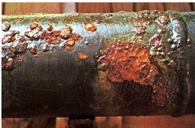
Figure 14.3 Pipe coating undercut by corrosion at small surface abrasions. (ref. 27).
