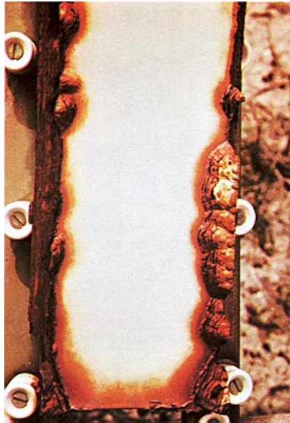
Figure 14.5 Edge corrosion on a painted test coupon in marine atmosphere. (ref. 29).
