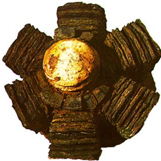
Figure 5.6 Exfoliation of steel nut on swimming pool fence. (ref. 10).
